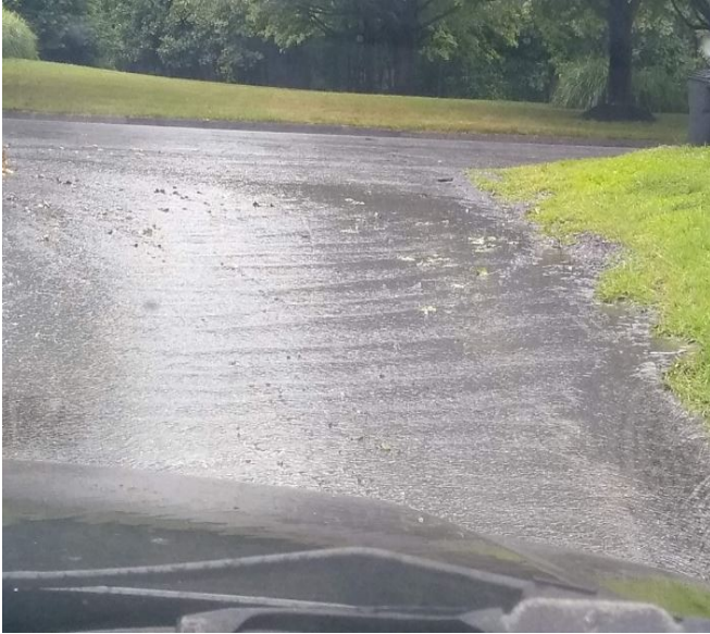
Before photo of stormwater pooling at the driveway entrance (2022).
