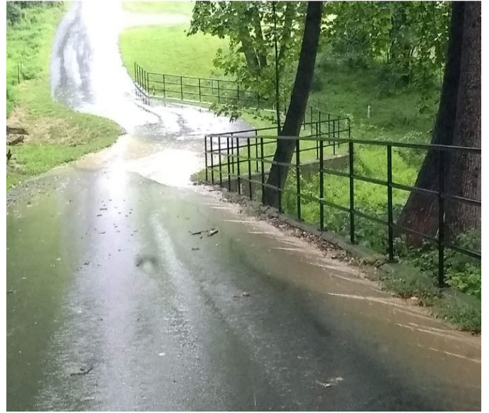
Before photo of stormwater pooling on street beside retaining wall (2022).
